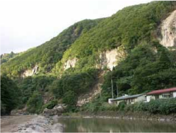
Photo 10. 湯湯付近に見られるトップリング（北川溶結凝灰岩中の節理の崩落による崩壊）。 Toppling failures occurred along Ichihazama river, because perpendicular joints are well developed in Kitagawa welded tuff. The photo was taken near Nuruyu hot spring.
